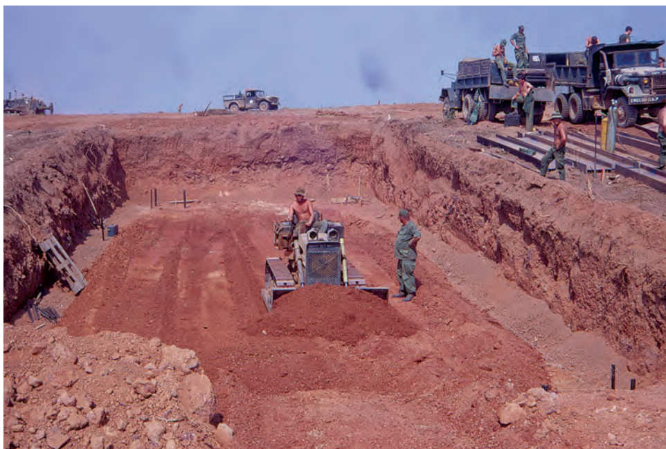
Excavating a tactical operations center at one of the new firebases north of Bien Hoa Air Base
